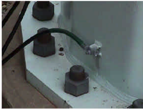
FIGURE 23-26 Example of Monopole Tower Ground Conductor
