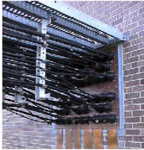
FIGURE 23-12 Intergraded Cable Entry Port with Ground Straps
