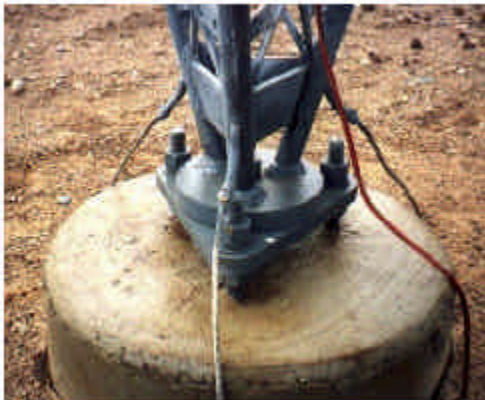
Figure 23-22 Guyed Tower Grounding
